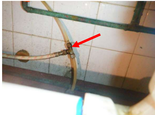
Water Leak Below Sink
