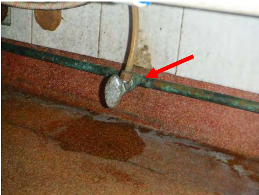
Water Leak Below Sink
