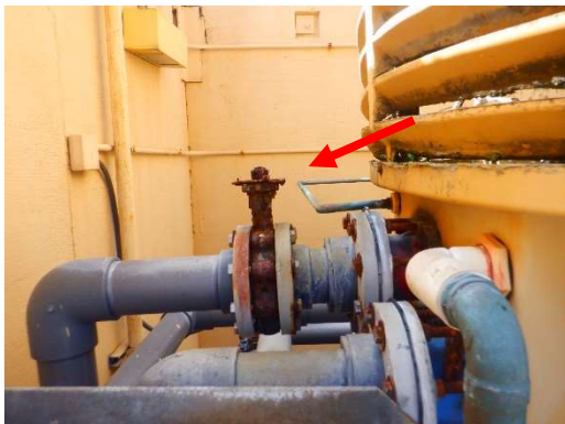
Corroded Valve Handles
