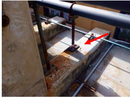
Corroded Pipe Stands
