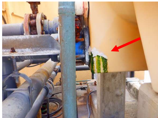
Crack Bottom of Chiller Housing
