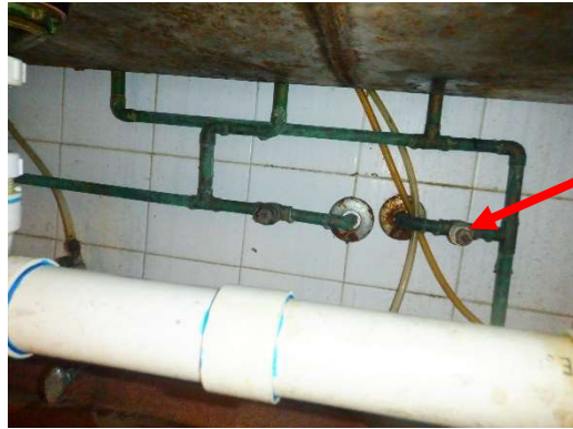
Missing Stem Valve Handles
