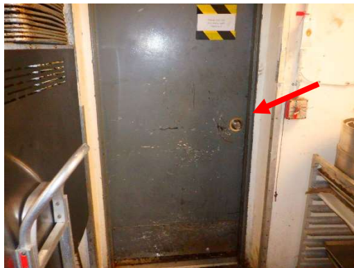
Incorrect Egress Hardware
