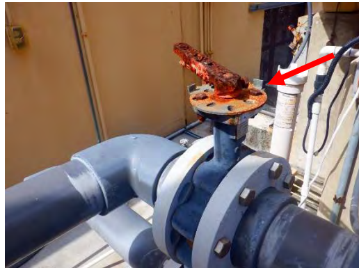
Corroded Water Valves
