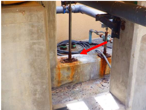
Corroded Pipe Hangers
