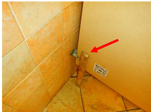
Bathroom Partition Not Secured
