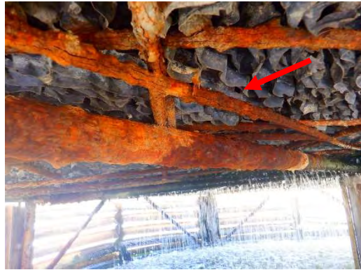
Corroded Pipe and Frame
