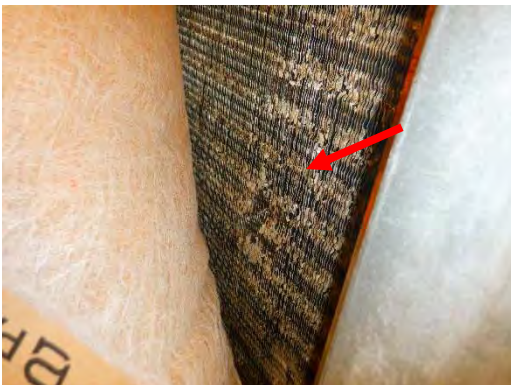
Brittle Heat Pump Coils
