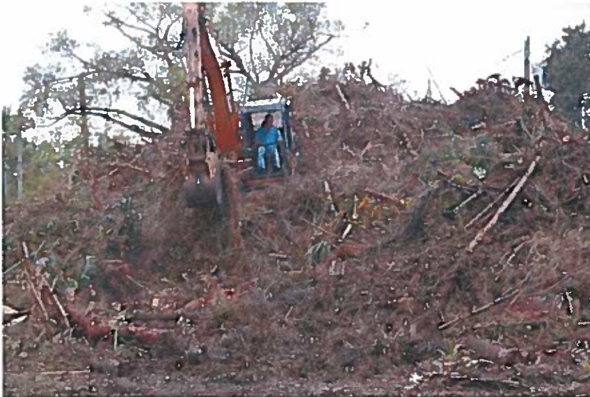
A worker in Biscayne Park operates a large excavator on top of a mountain of debris. Emily Michot - emichot@miamiherald.com
