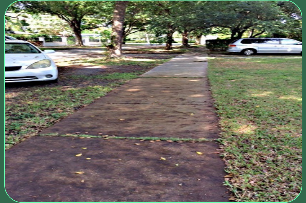
5 = Severe and Objectionable staining
