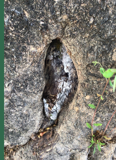
Areas of decay or cavities
